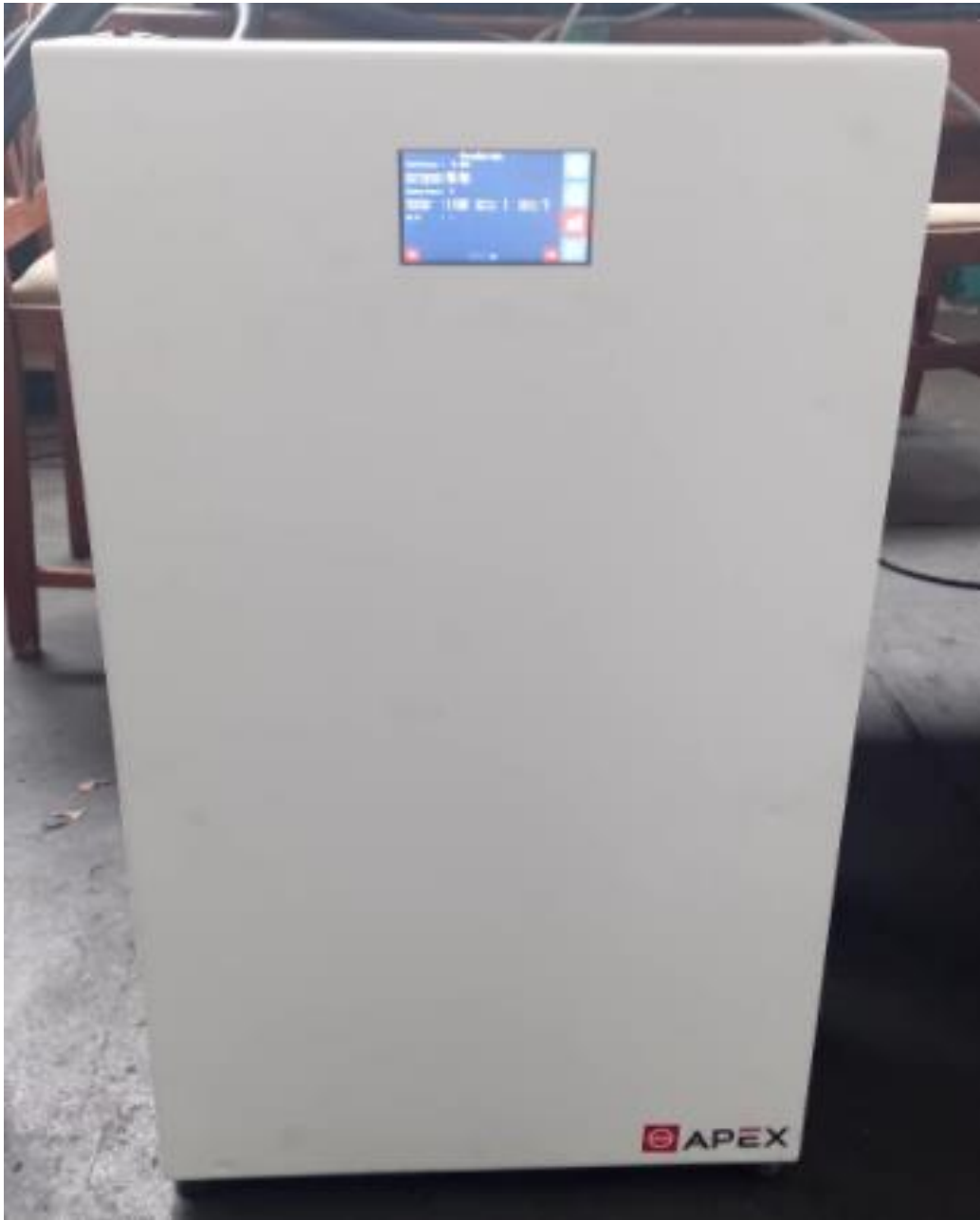
Commercial 10kWh battery with inhouse built BMS
